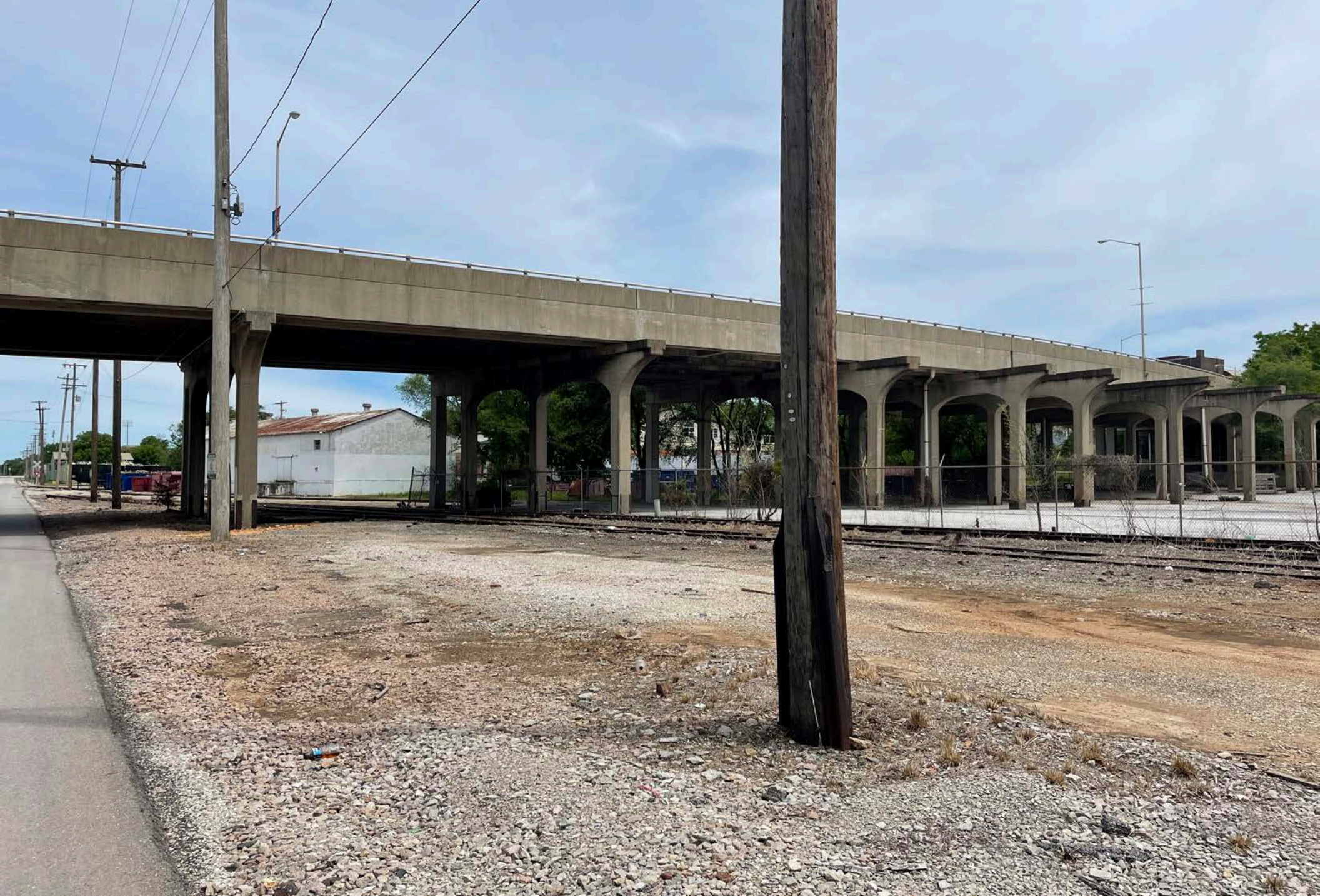
Figure A.11 East Phelps Street looking east at North Benton Avenue bridge
